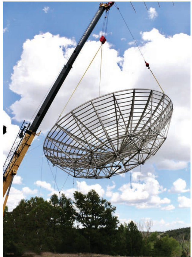
The dish lifted in the air by a crane and rotated to the birdbath position while being lowered to the ground.
