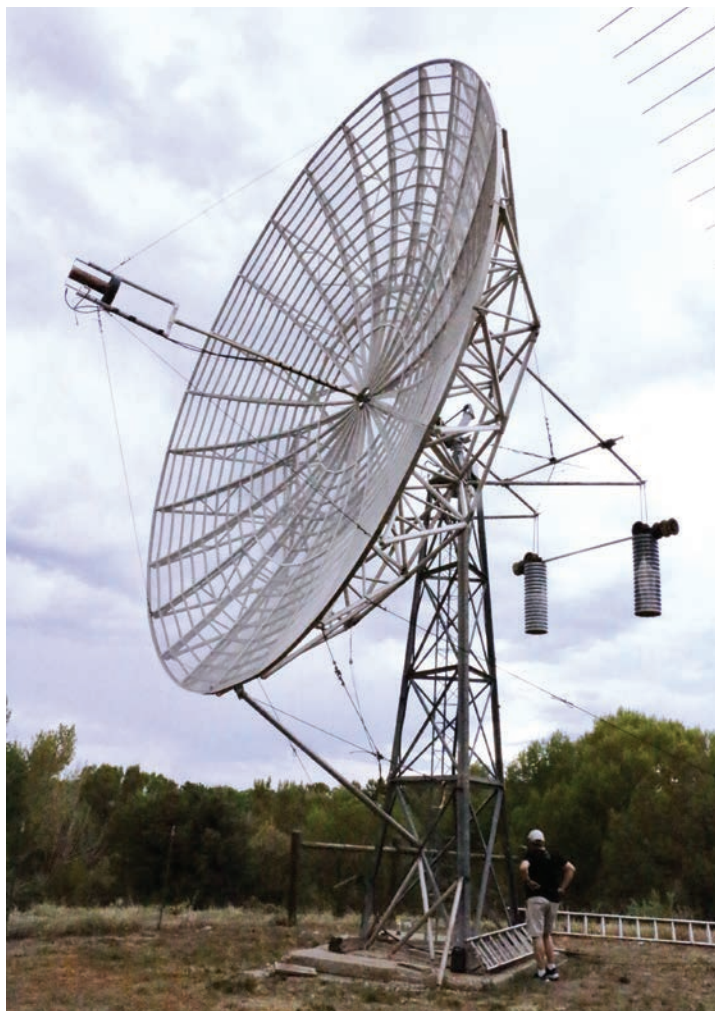
The 30-foot dish in the sideways position. This position presented the first challenge to the crew and the crane operator.
