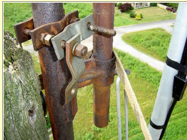
The curved clamps at left are ready to accept the mast with feedlines on the right. There was very little wind so raising the 20 foot mast and clamping it in place was not a problem.
