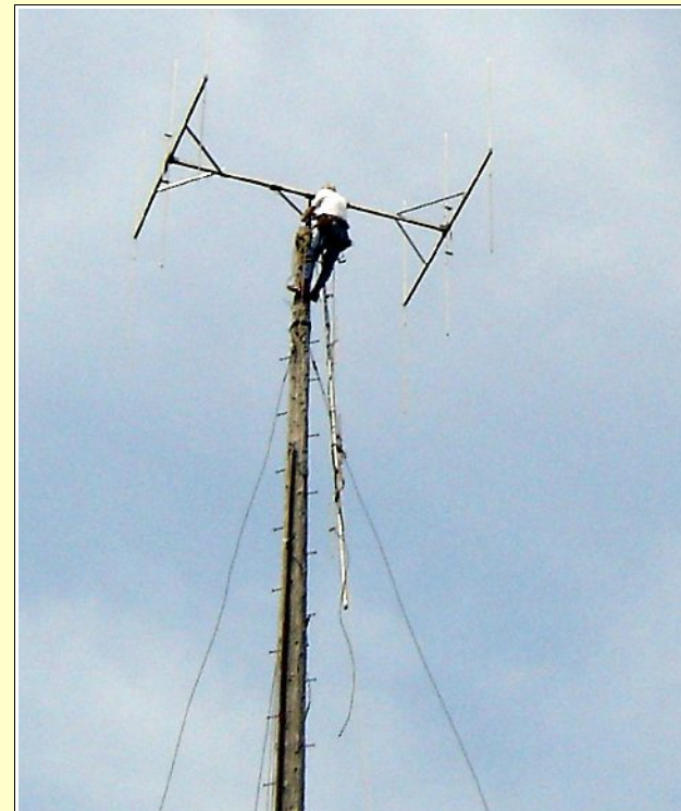
Pete WW30 prepares to install the 4-bay Antenna Specialist antenna at the top of the 100 foot cedar pole. An old pair of low-band yagis will be removed later.
