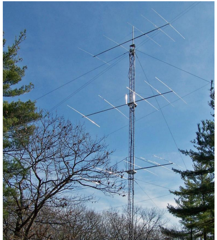
Figure 5 - Part of the antenna farm at K1WHS. This is the rotating 5/5/5 stack. (Photo - K1WHS)
